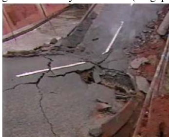
Fig. 2 Sudden collapse of Ynys-Y-Gwas bridge (UK, 1985)
