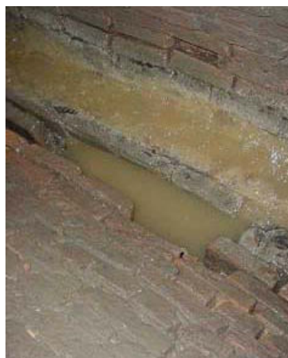
Fig. 7a Deterioration of the bottom of the sewerage canalisation by the velocity of water.
