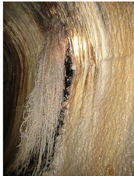
Fig. 12 Obstruction and fissuration of the canalisation by vegetation (weak maintenance).
