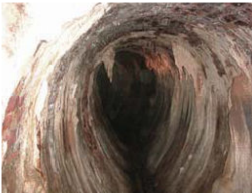
Fig. 9 Obstruction and reduction of the diameter of canalisation of the drainage by sedimentation (weak maintenance)
