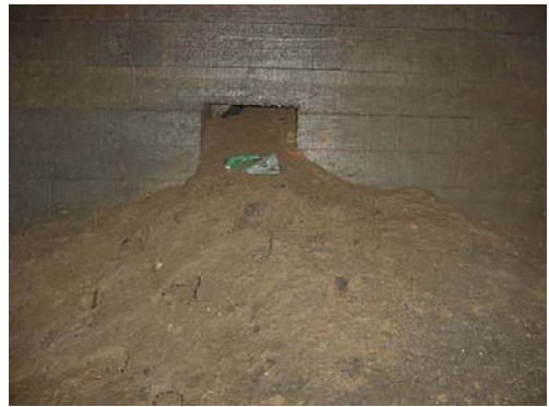
Fig. 11 Obstruction of the canalisation connection by old mud deposits (weak maintenance).
