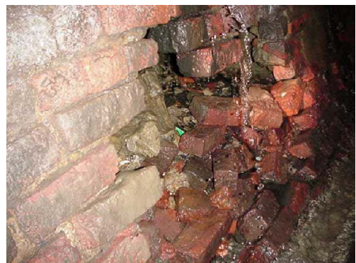
Fig. 13 Destroy of the wall of culvert by the water pressure (Absence of pore drainage in the wall: weak maintenance).
