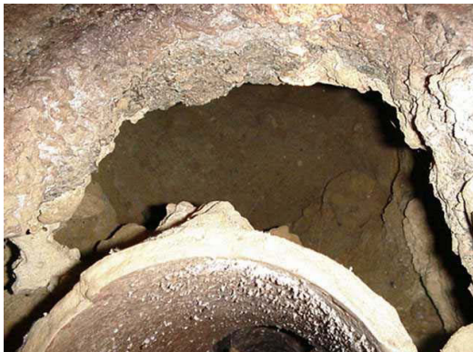
Fig. 10 Delamination of the canalisation by the flood.
