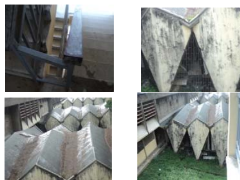
Fig. 1 Corrosion attacks of steel and concrete structures in the University of Lagos, Nigeria
