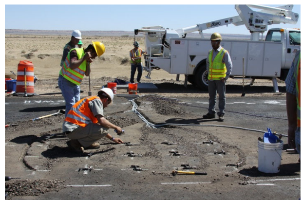
Fig. 3 Installation of horizontal strain gauges
