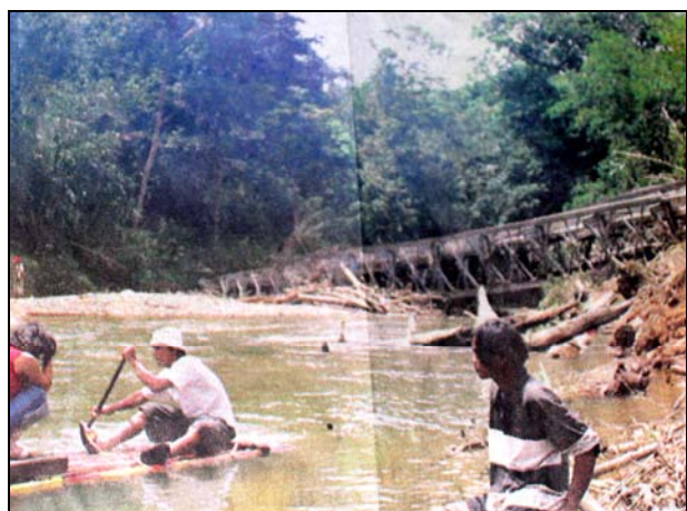
Fig. 8 Bailey bridge collapse due to heavy floods [20]
