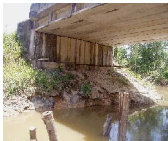
Fig. 5 Bridge failure due to scouring at Bokah Rasau Stungkor Road, Kuching, Sarawak [20]
