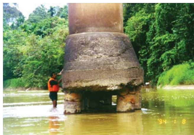
Fig. 4 General scouring of river bed at Sg. Jeniang, Kedah
