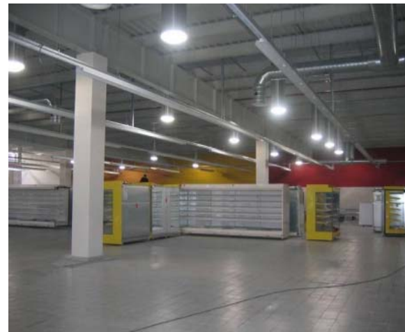
Fig. 3 Storeroom illuminated by light pipes
