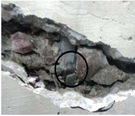
Fig. 5the necking phenomenon of steel strips
