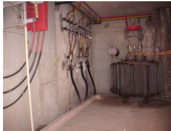
Fig. 2 Magnetic field measurement at distribution substation
