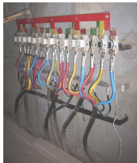
Fig. 3 Low voltage panel view
