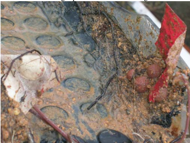
Fig. 6 Roots seemed to have grown into the liquid applied waterproofing at the edge
