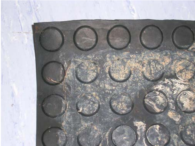
Fig. 9 Clean sheet membrane edges indicate no form of growth between the liquid applied waterproofing and sheet membrane
