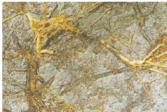
Fig. 1 Roots leaving impression on waterproofing membrane, adapted [10]
