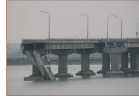
Fig. 18 Case 2: the bridge failure in flood
