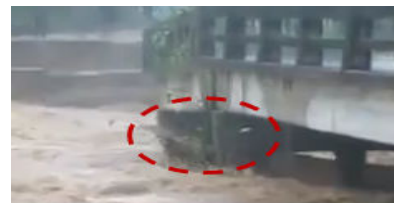
Fig. 19 Case 3: the bridge failure in flood
