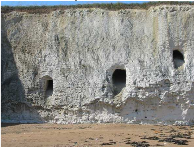
Fig. 3 Cavities of typical piping / sapping erosion [6]
