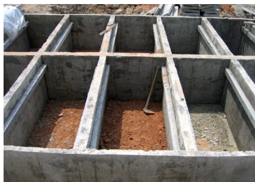
Fig. 20 Picture shows the use of pre-cast concrete at Subang Lutheran Garden (Lei Wei Min)
