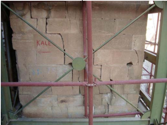
Fig. 2 Close view of the middle gate entrance wall on the valley side
