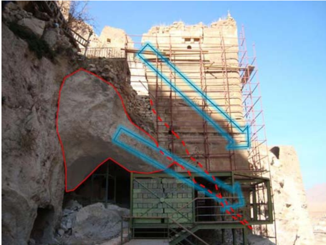
Fig. 1 Middle Gate general view, cracked rock & force paths, and crack pattern
