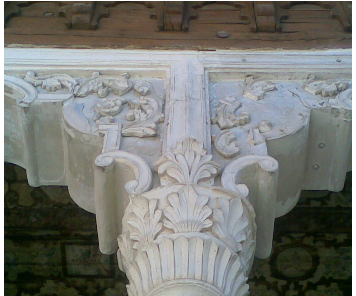
Fig. 3 Damage to the historic building of temperature and humidity changes
