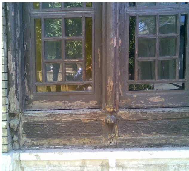
Fig. 5 Decomposition of Wooden door – Ghavam House -Shiraz Esfehan
