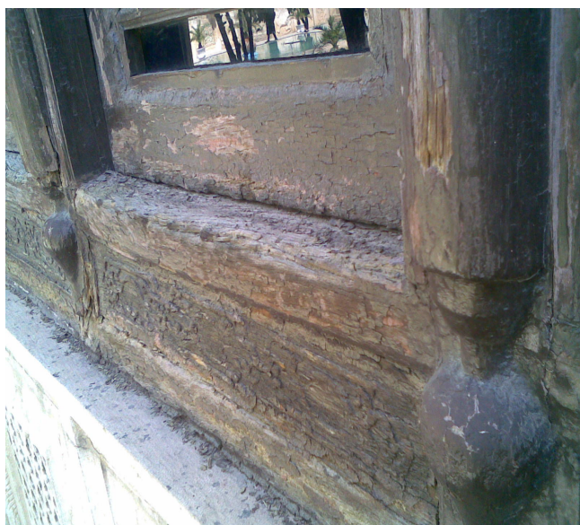
Fig. 4 Decomposition of Wooden door – Ghavam House -Shiraz Esfehan
