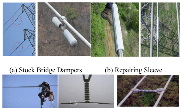
(a) Stock Bridge Dampers (b) Repairing Sleeve (c) Performed Armor Rods (d) Spacer Fig. 3 Obstacles on transmission line
