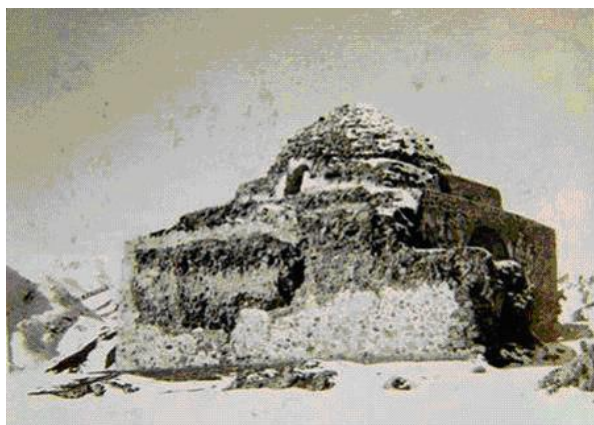
Fig.38 An image of eastern wall of cross-vault "Baze-hur" before mending and the hole created on it
