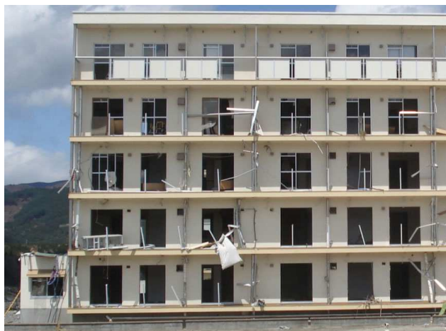
Fig. 18 Detail of damages on balconies
