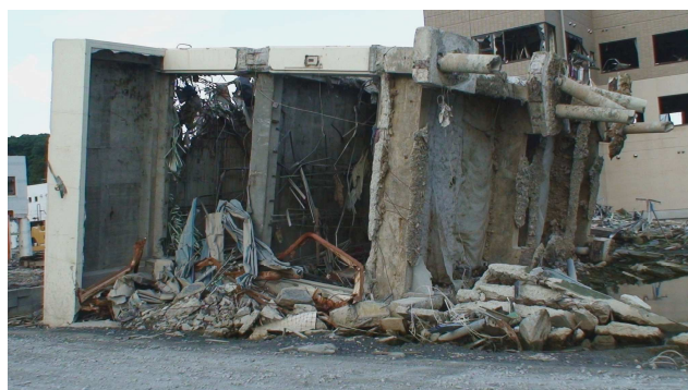
Fig. 23 Collapse of 2 story RC building
