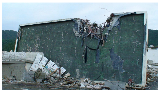
Fig. 24 Detail of impact on the building
