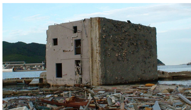
Fig. 22 Detail of slab foundation of collapsed building
