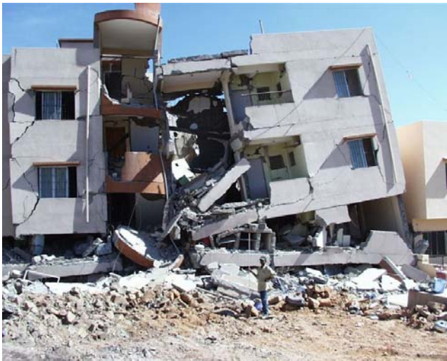
Fig. 1. Example of a horizontal layer with survival space in the collapsed first floor. Photo: Michael Markus.
