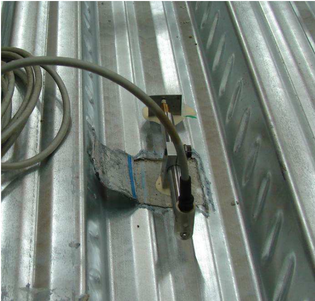
Fig. 5 Configuration of the measuring device for monitoring sliding on the interface between the concrete and the steel sheet
