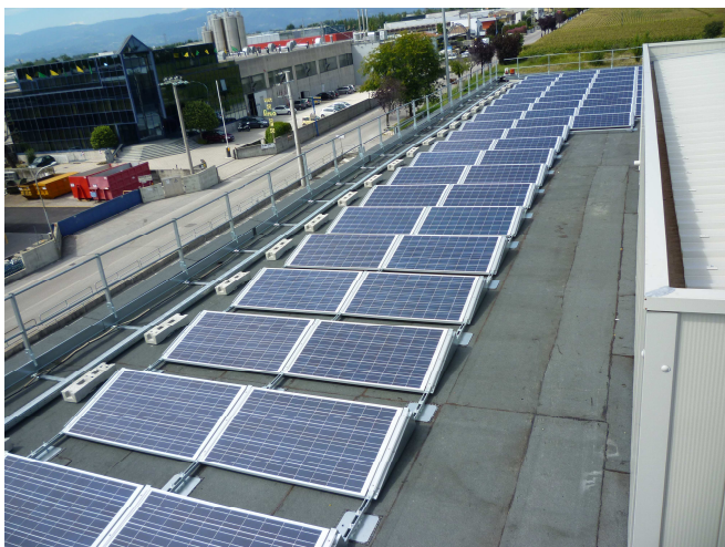
Fig. 5 Displacement of the PV panels on the top of the SMART centre
