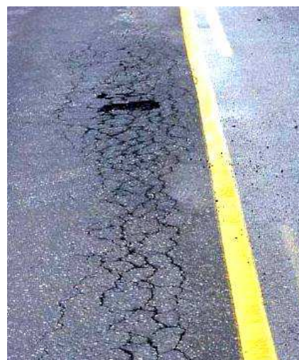
Fig. 4 fatigue causes pothole
