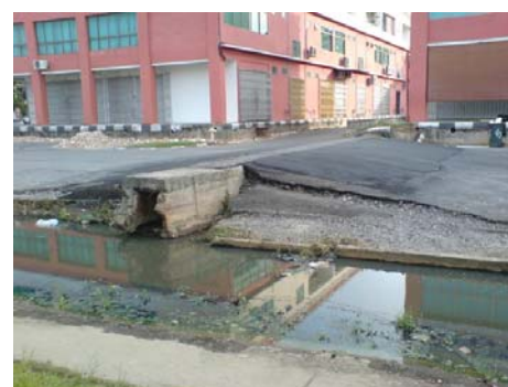
Fig. 2 Ground settlement caused poor drainage and road system in a commercial lot, Sibu.
