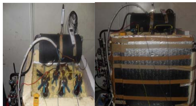
Fig. 9. The transformer measurements.
