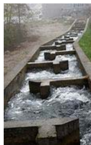
Fig. 2 By-pass device as designed fish passage
