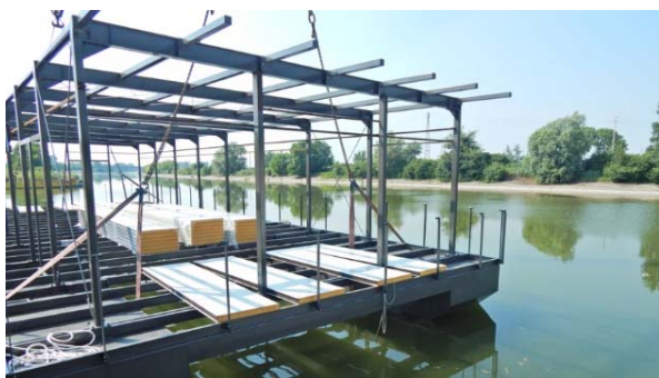
Fig. 8 Metal structure during construction of Tintero Boat Restaurant (Photo by Giancarlo Battilani and Minimal) [17]
