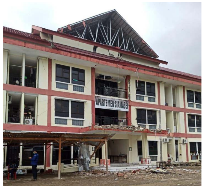
Fig. 2 (b) Damage to a building ( Asrama Polsek Mamuju ) due to the Mamuju earthquake on 15 January 2021 [4]
