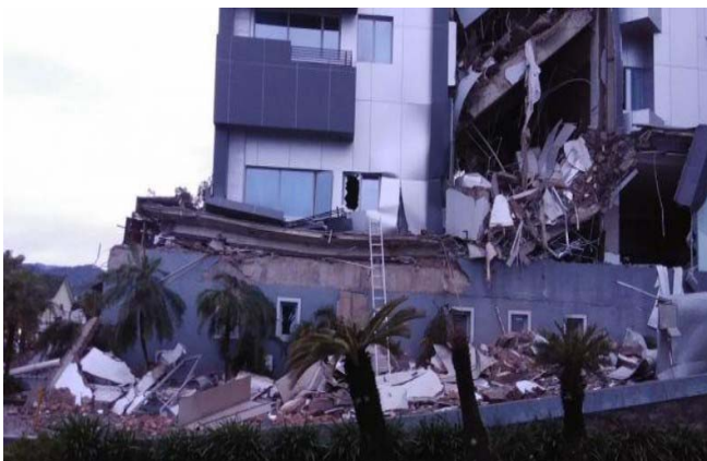
Fig. 2 (a) Damage to a building ( Hotel Maleo Mamuju ) due to the Mamuju earthquake on 15 January 2021 [4]
