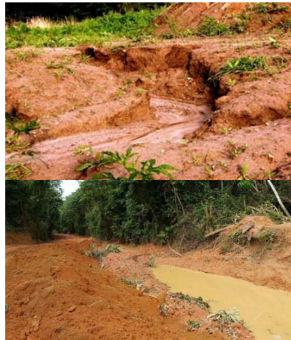
Fig. 1 Fluvial Erosion in Construction/Mining Areas
