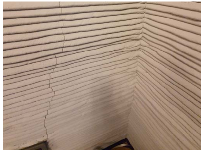
Fig. 1 Crack in the dry mortar wall
