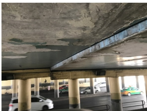
Fig. 7 Height difference of capping beam
