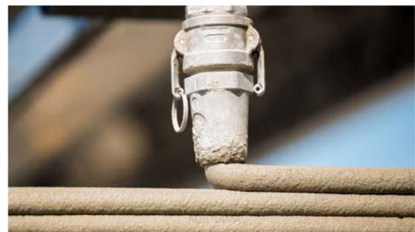
Fig. 2 Icon's Vulcan construction system 3-D prints layer on layer using specially formulated concrete [11]
