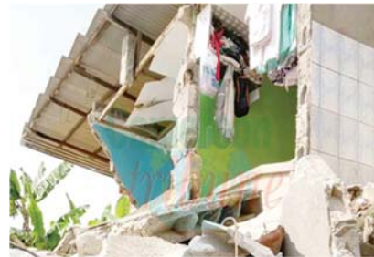
Fig. 2 Collapse of one storey building in the Ndogbong suburb
