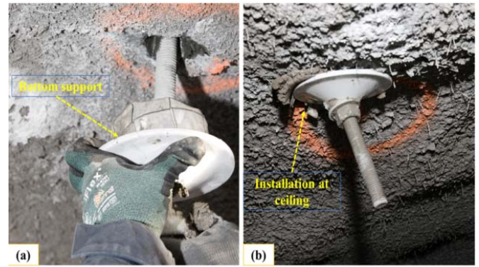
Fig. 15 Application of pucks on the tunnel ceiling a) during installation process, b) after installation of puck
