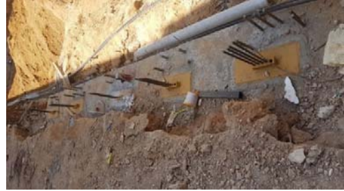
Fig. 4 Piles in Section 1 with prestressing strands added to the conventional reinforcement structure
