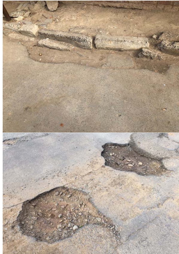
Fig. 7 The potholes on R37 roads
