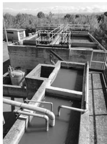
Fig. 1 Wastewater treatment plant
