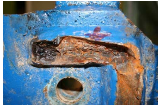
Fig. 1 Joint n. 2. Fracture surfaces covered with rust
