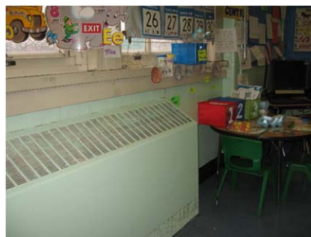
Fig. 2 Classroom with perimeter radiators at Elementary school in Bronx, NY 2012 [5]
