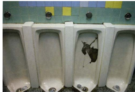
Fig. 6 Urinals in Poor Condition at Elementary School in Brooklyn, NY [5]
