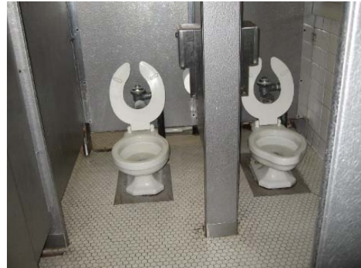
Fig. 5 Toilet Stall Doors Removed at School in Brooklyn, NY [21]
