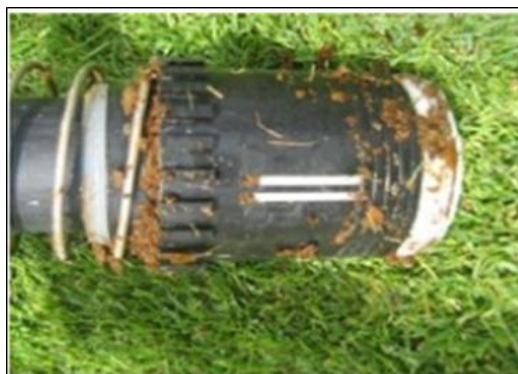
Fig. 2 Sprinkler clogged by scale
