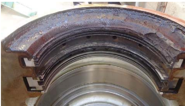
Fig. 7 Heavy coke deposition, rubbing marks on Bearing#01 housing
