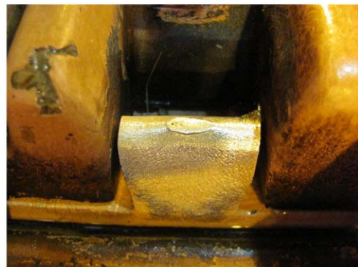
Fig. 11 Damaged copper contact in an equipotential dogbone busbar
