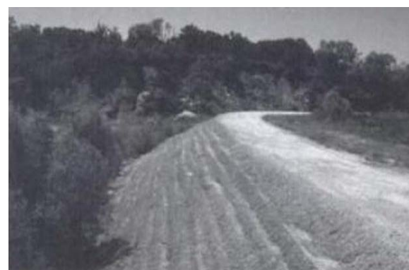
Fig. 8 RCC stepped spillway of Brownwood County Club dam after 6 times of overtopping.
