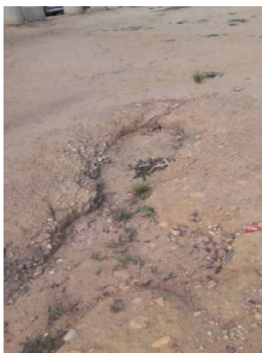
Fig. 3 Erosion in the area
