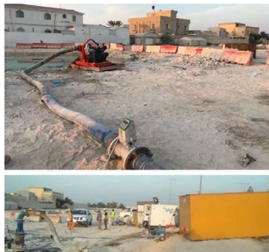
Fig. 22 Water pumped into the injection well from EFA pond at Site 10, FPS14
