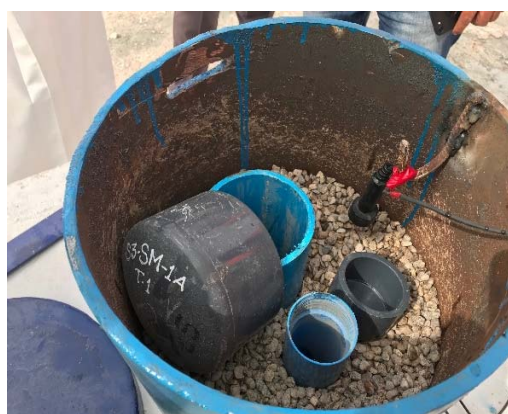
Fig. 15 Top view of shallow monitoring well
