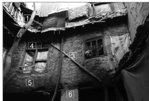
(a) A traditional type of house: 1 – Wooden parapet, 2 – Mud roof, 3 – Adobe wall (Sinj construction), 4 – Wooden window, 5 – Mud–straw plaster, 6 – Adobe column
