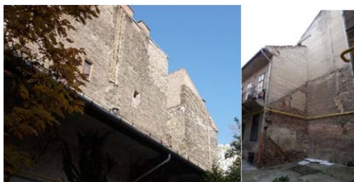
Fig. 5 Two of the many empty firewalls in the case study that could be used as green walls
