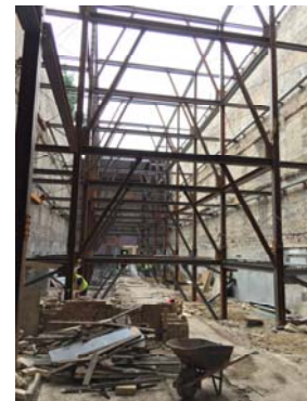
Fig. 19 Newly installed structural steel frame. Portion of old brick wall is still visible in the foreground
