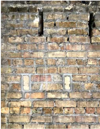
Fig. 20 The very rough inside face of an existing perimeter three-wythe thick masonry wall, with as-yet-to-be filled joists pockets
