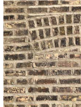
Fig. 22 Southern-facing former window opening, with toothed-in flush in-fill brick; this modification was done sometime prior to the conversion of the apartment building into a museum
