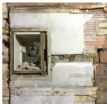
Fig. 6 An uncovered milkman delivery door, leading to center communal corridor. This has been sealed over for decades
