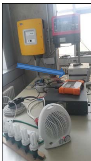
Fig. 3 (a) Inverter grid-connected test circuit (b) Schematic diagram of Inverter grid-connected test circuit
