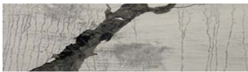
Fig. 1 Fibres stitching of a diagonal crack
