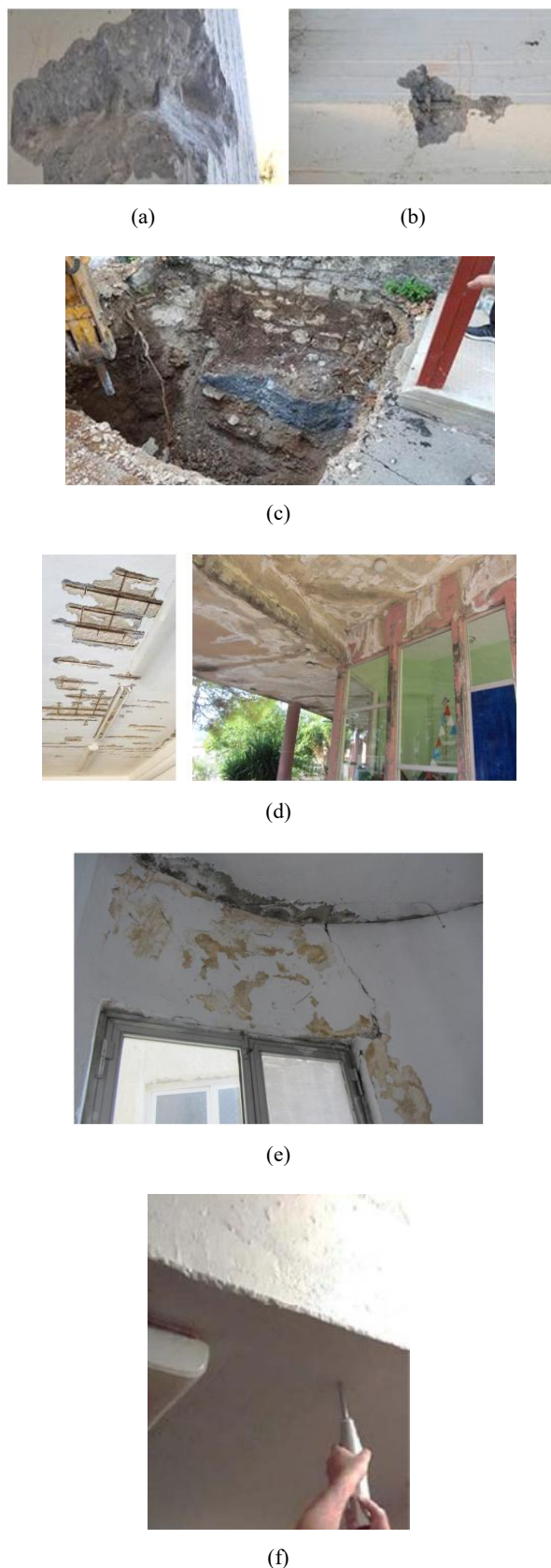
Fig. 3 Disclosure of steel reinforcement materials (a,b), disclosure of the foundation in a column (c), localized damage (d,e), and a non-destructive test (f)
