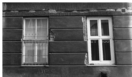
Fig. 3 Disagreeable modernization of a window by neglecting historical values (photo of Attila Zsoldos BSc Architect student)
